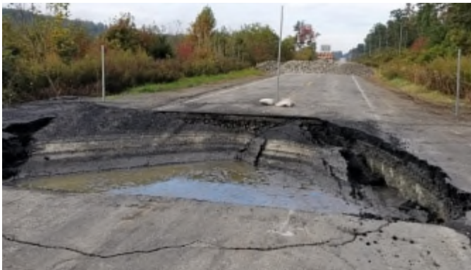
Figure 4.3.7-1. Sinkhole in Porter Township, October 2017
