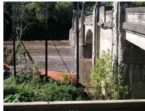
Flooding in Manayunk during Hurricane Ivan
