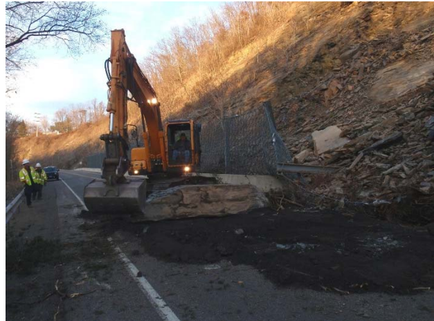
Landslide on St. Rte. 4012, January 2016
