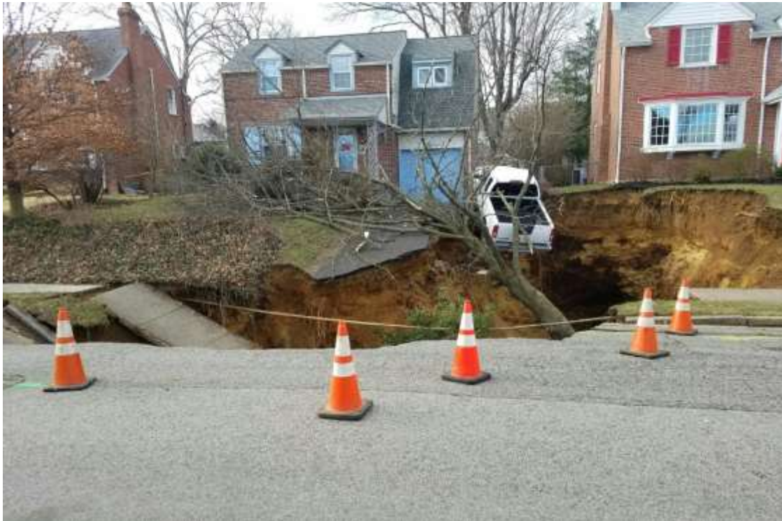
Sinkhole at 720 and 724 Brooke Road
