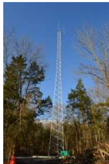
Emergency Communications site in Upper Frederick
