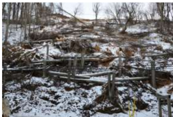
Landslide above Balligomingo Road
