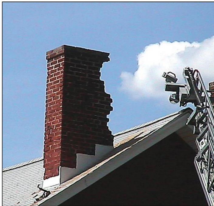
Figure 4.3.4.3.1: Chimney Damage (Fayetteville, PA) - Aug 2011 Earthquake 35
