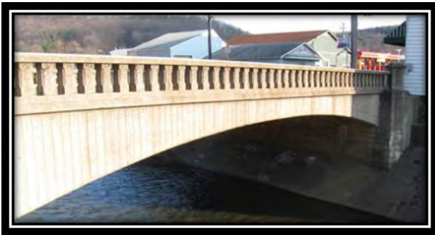
Figure 4-51: Pennsy Bridge before collapse.
