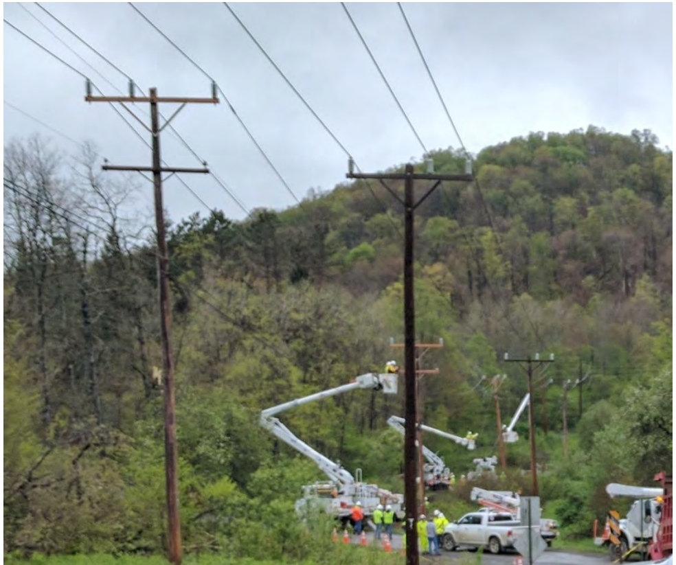
Figure 28-West Penn Power responding to lines down in Jones Township after tornado blew through the area in May of 2017.
