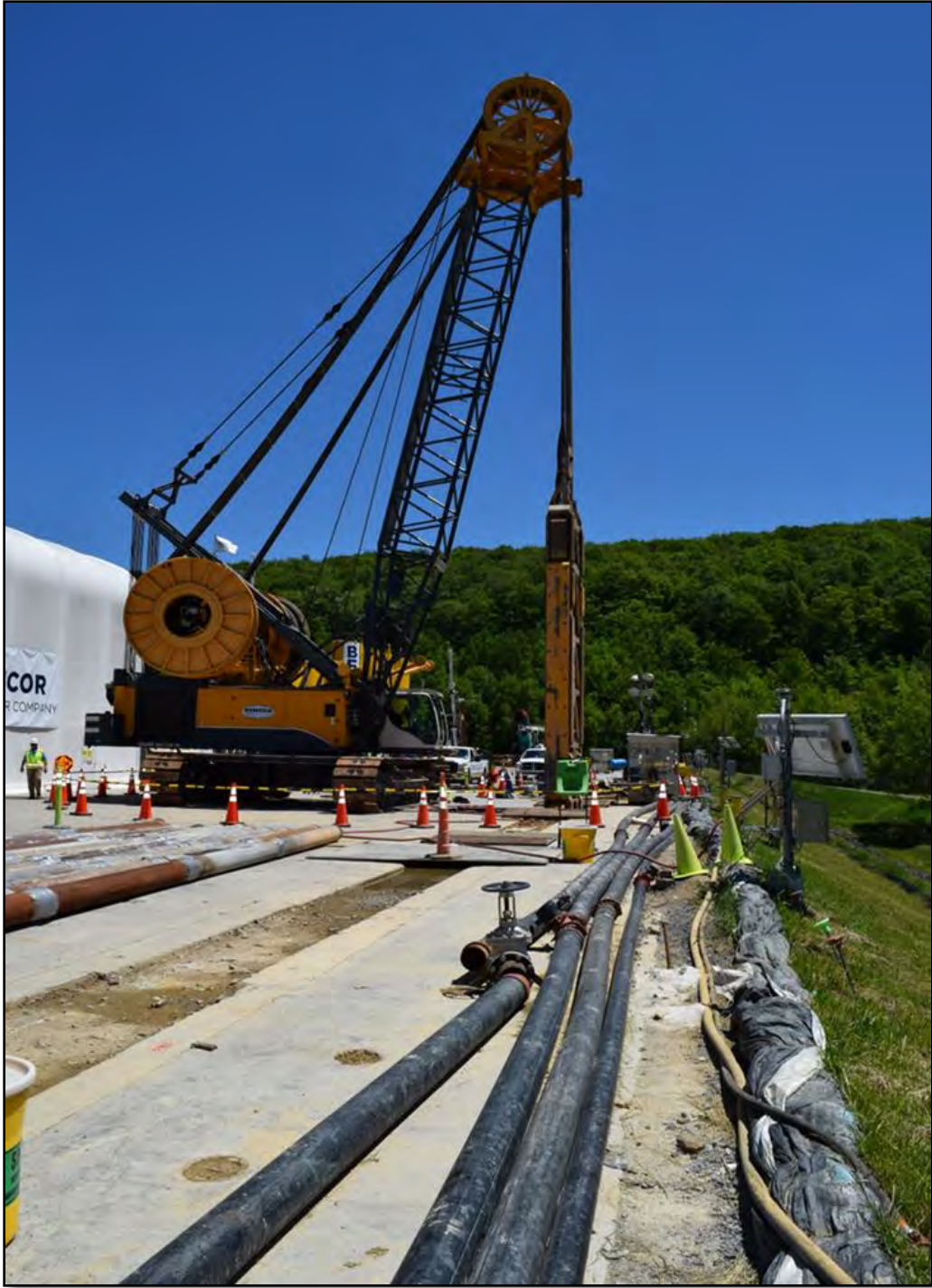
Figure 4-4: Drilling into the East Branch dam wall. Photo courtesy of the US Army Corp of Engineers
