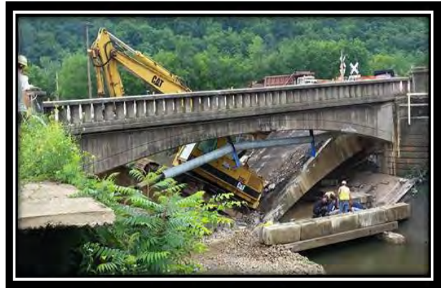
Figure 4-52: Below- The Pennsy Bridge on Route 219 after a partial collapse. A Clarion PA company was fined for serious violations
