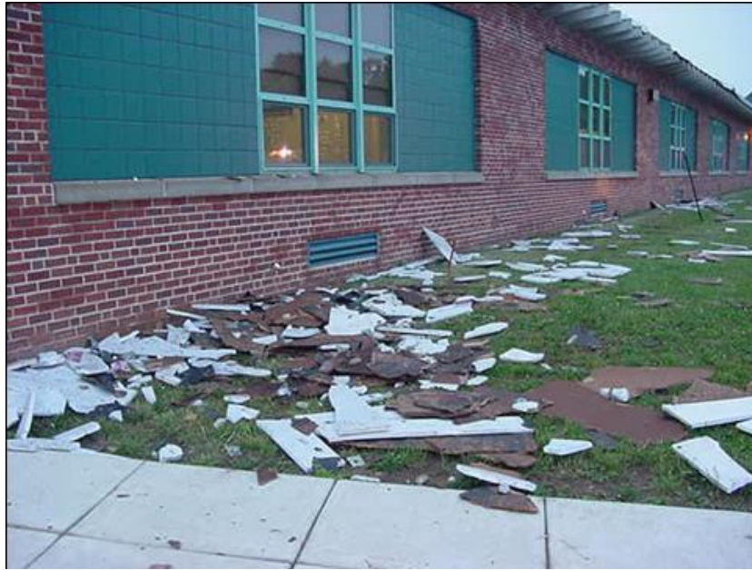
Figure 4.3.7-1: Straight line wind damage at WG Rice Elementary School in South Middleton Township, Cumberland County, PA in July 2000 (Photograph courtesy of Cumberland County, 2014).
