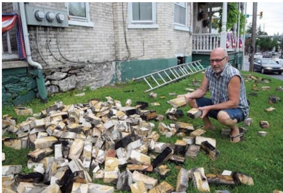
Figure 4.3.2-2: Earthquake damage (collapse of brick chimneys) in Mount Holly Springs, Cumberland County, PA on August 23, 2011 (Photograph courtesy of Jason Malmont/ The Sentinel , 2014).
