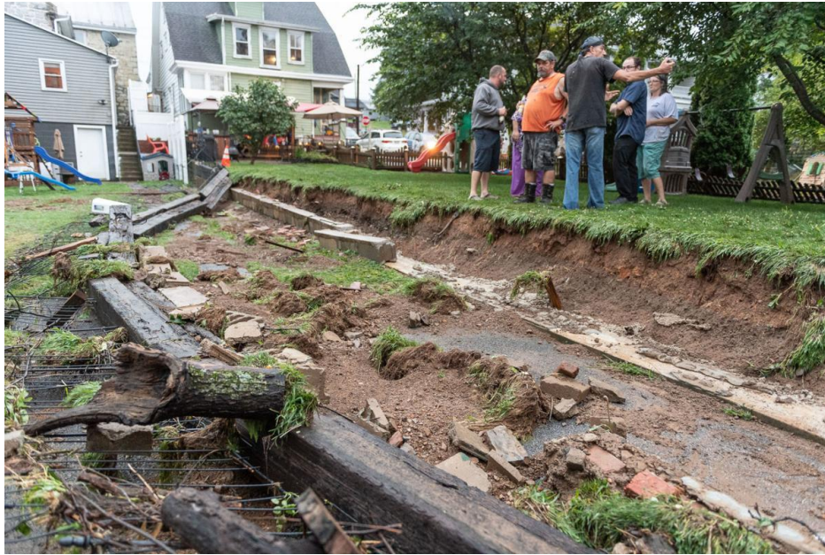
Figure 4.3.3-6: Damage to a retaining wall caused by excess stormwater in Newville, PA (Photograph courtesy of Wes Peterson, The Sentinel , 2018).
