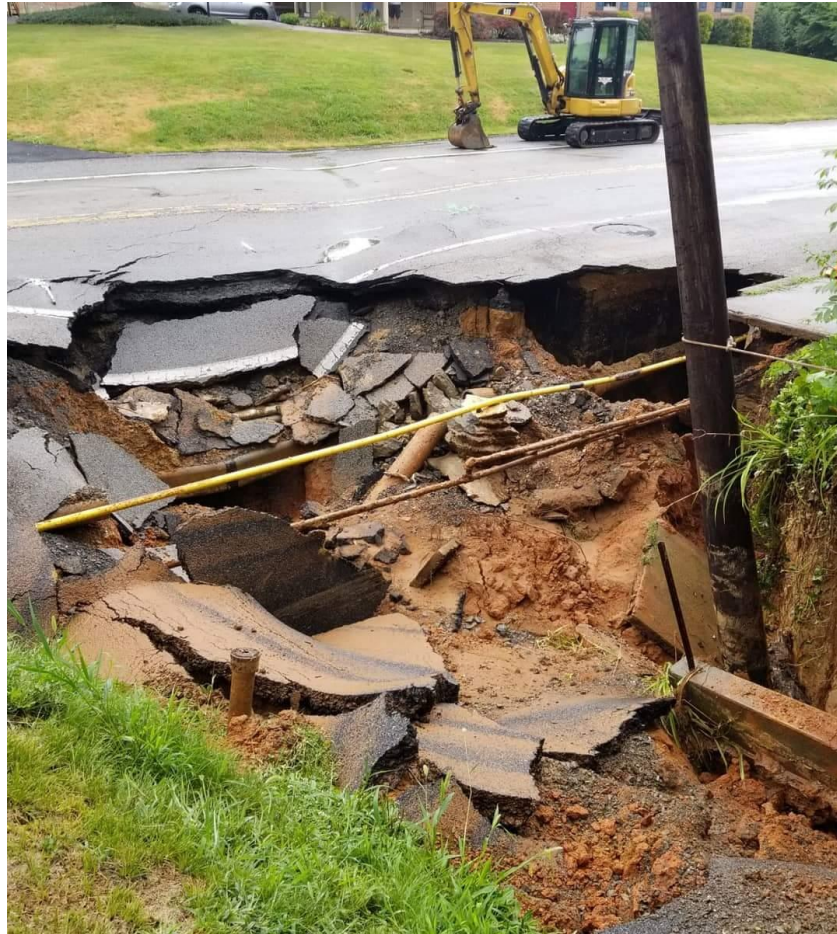
Figure 4.3.6-3: Sinkhole along a Cumberland County Roadway (Photograph courtesy of Cumberland County Department of Public Safety).
