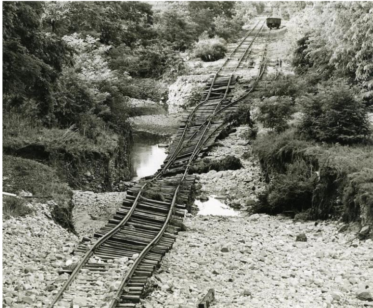
Figure 4.3.4-2: Flood damage to the Reading G&H Branch at Carlisle Junction (Cumberland County, PA), due to Hurricane Agnes (Photograph courtesy of Michael Bupp/ The Sentinel , courtesy of the Cumberland County Historical Society, 2018).
