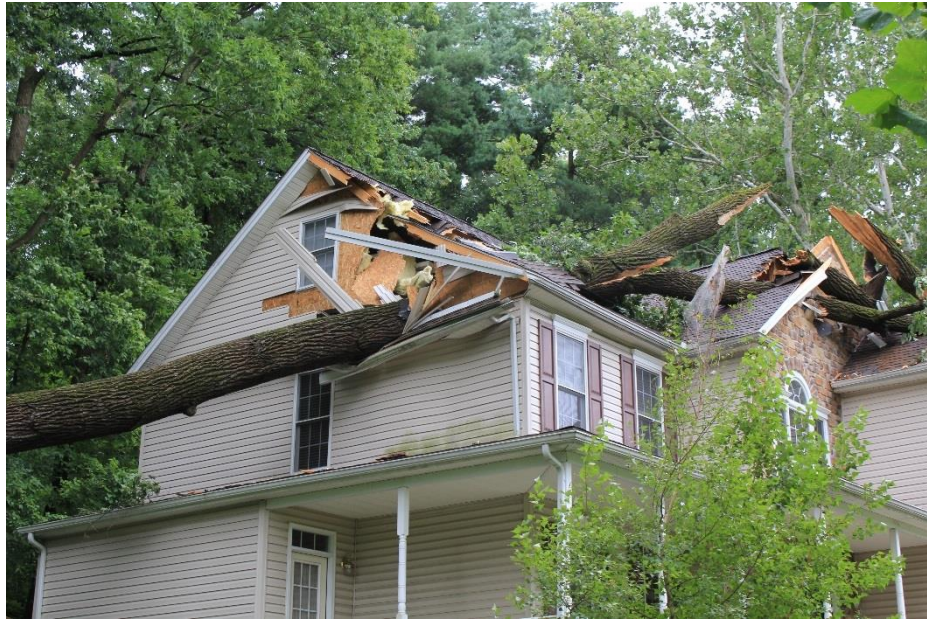
Figure 4.3.4-1: Hurricane Irene damage to a residence in Lower Allen Township, Cumberland County, PA on August 28, 2011 (Photograph courtesy of Lower Allen Township, 2014).
