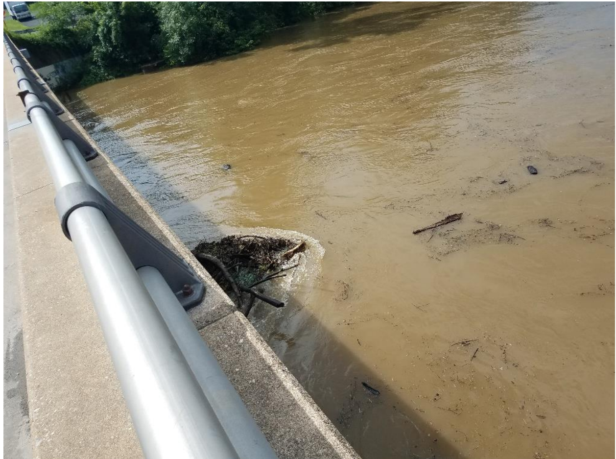
Figure 4.3.3-5: Obstruction of a bridge with debris in East Pennsboro Township (Photograph courtesy of East Pennsboro Township).
