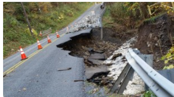
Figure 4.3.6-3: Road Failure Along Purdue Mountain Road in Benner Township, 2016 (Benner Township, 2018)
