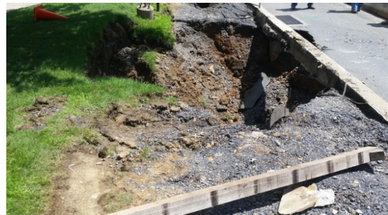
Figure 4.3.10-3: Sinkhole on Bigler Road on Penn State’s campus (Murach, July 2015b)
