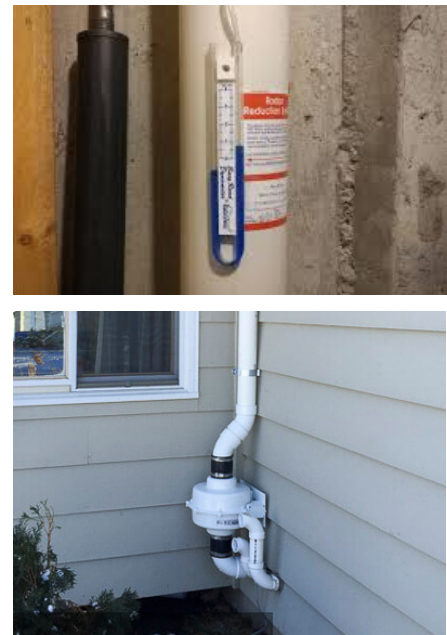
Figure 4.3.8-7: Radon Mitigation Systems (Scott Home Inspection, 2017) (IRadon, 2020)
