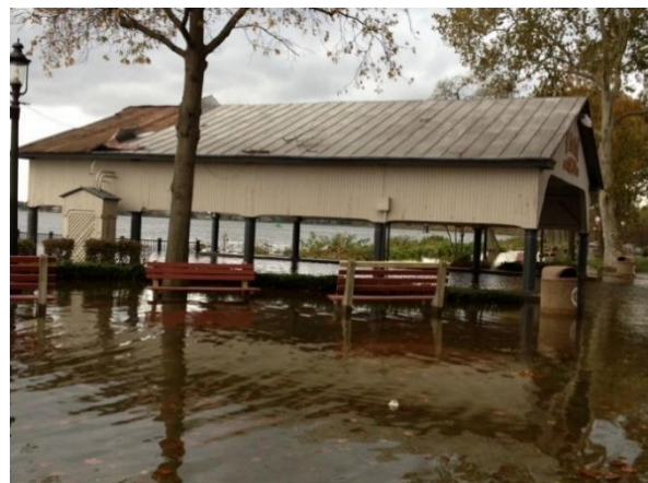
The Bristol Wharf experienced flooding and roof damage.
