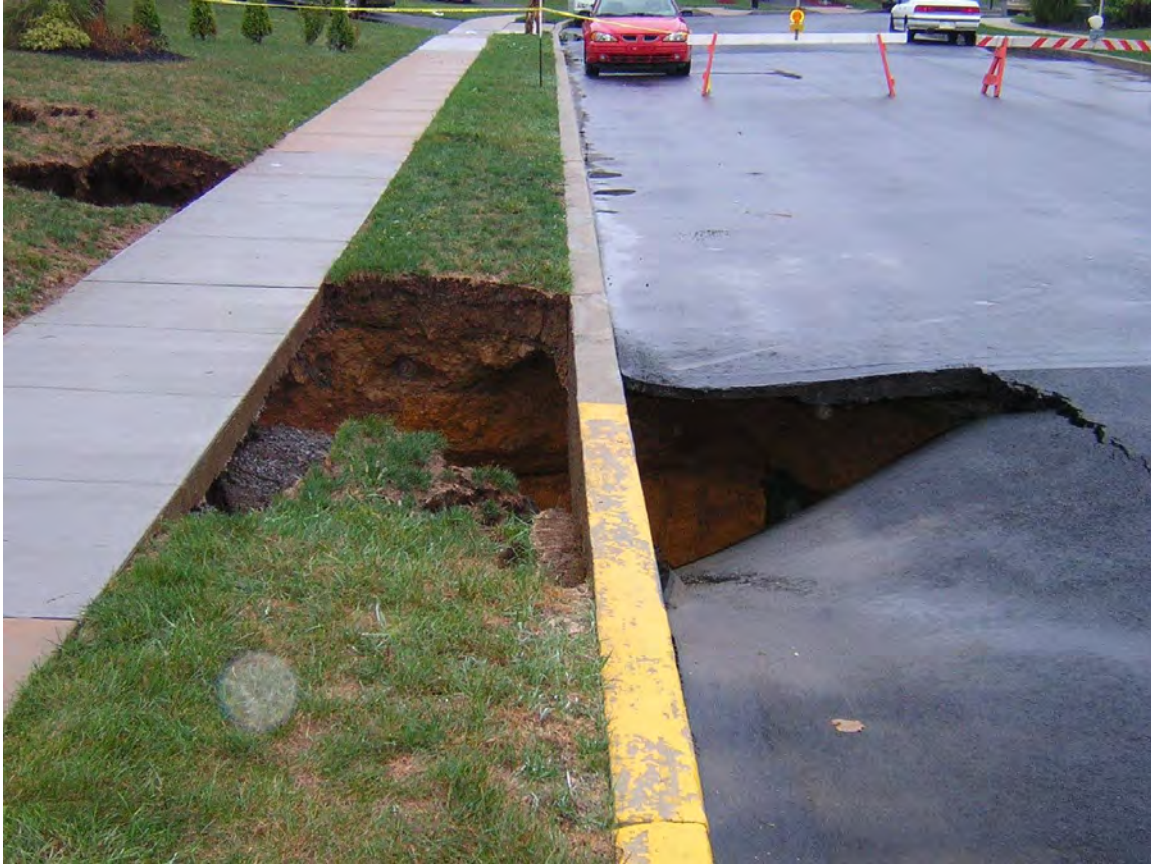
Sinkhole in Sinking Spring Borough
