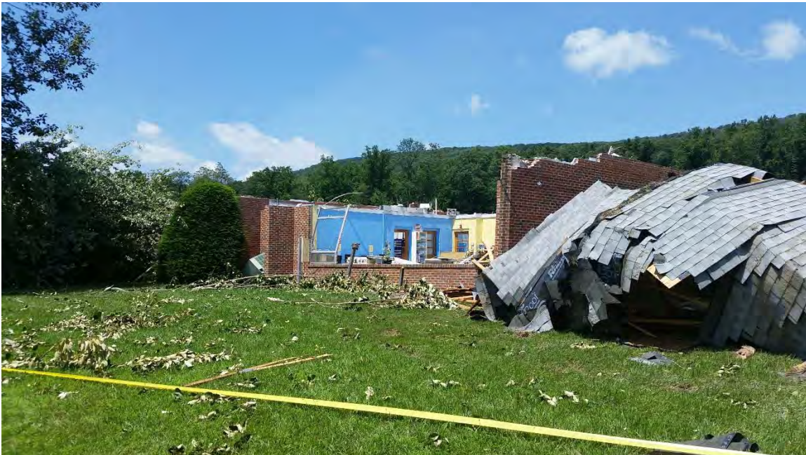
2015 Tornado Damage to the Blue Mountain Elementary School
