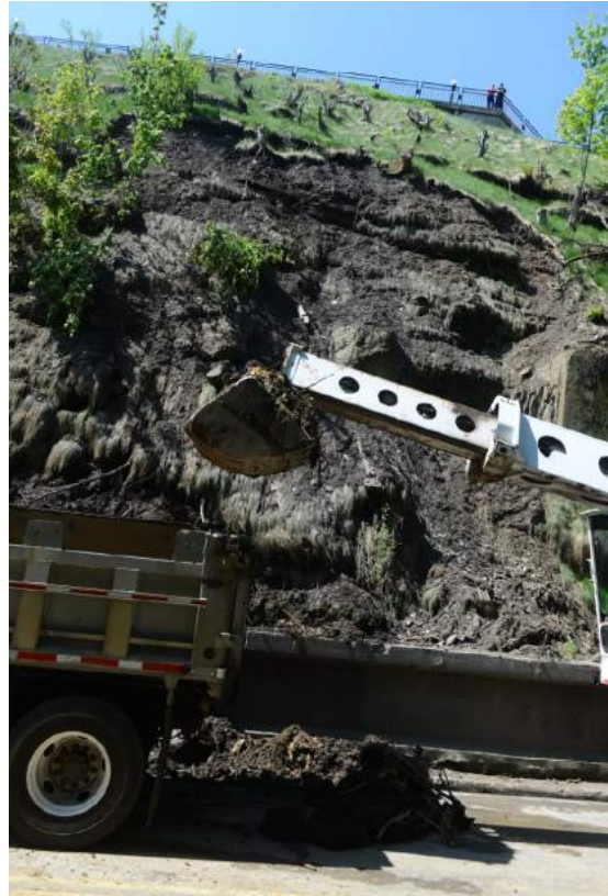
2014 Landslide Damage on PJ McArdle Roadway.
